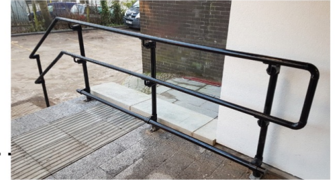
DDA Compliant Handrail
