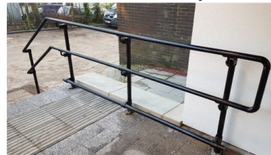
DDA Compliant Handrail
