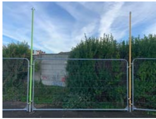
Demountable Heras fence panels and steel posts
